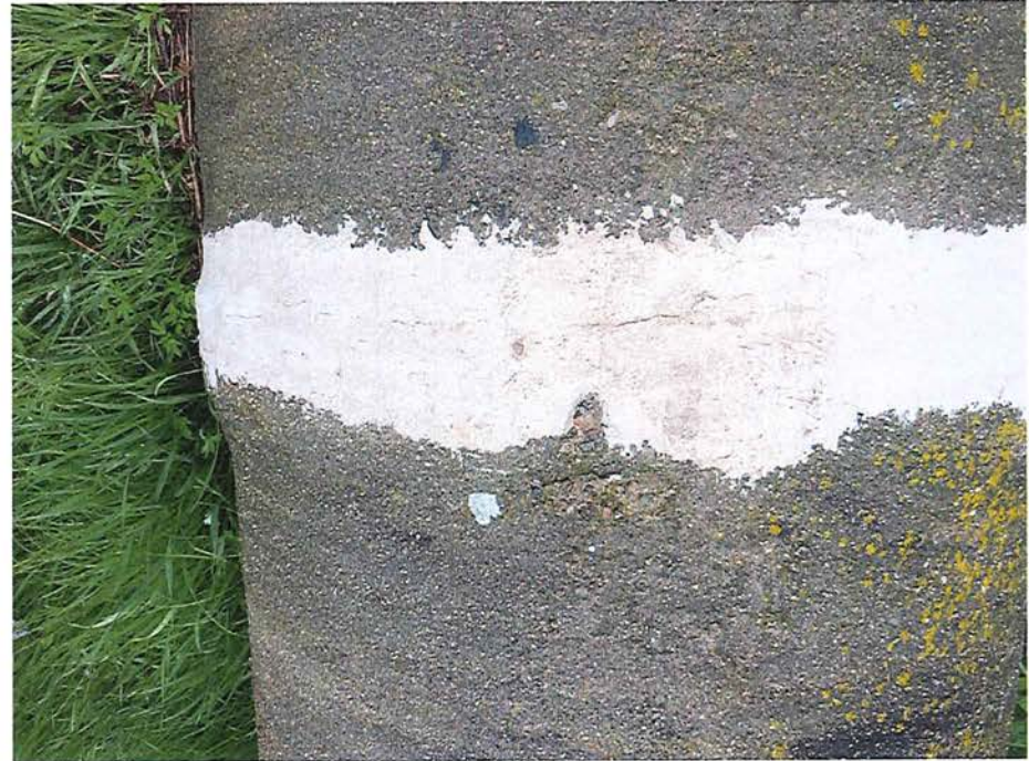
1 st Joint of Outlet – small crack in epoxy
