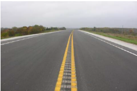
Centerline Rumble Strips Source: Mitigation Strategies for Design Exceptions (FHWA, FHWA-SA-07-011)
