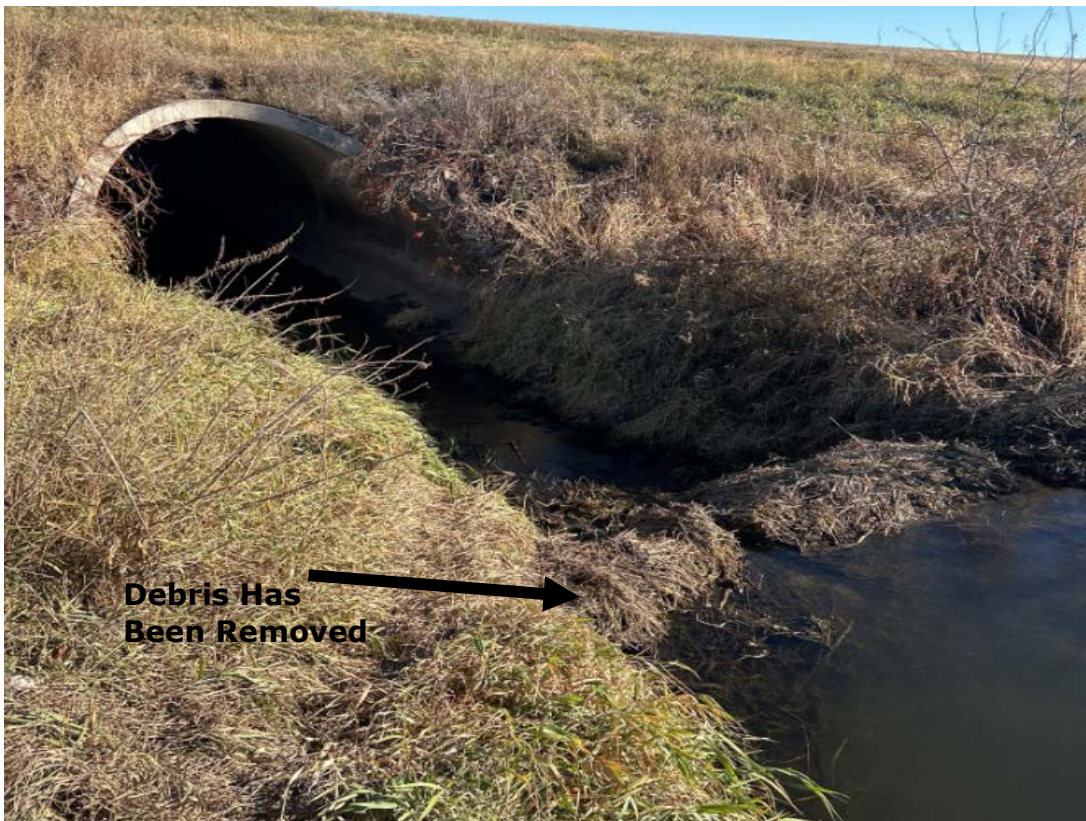
Figure 8. CD 12 Terminus into Rice Creek at CSAH 6 (NE \frac{1}{4} of SE \frac{1}{4} of Section 7 of Delhi TWP)
