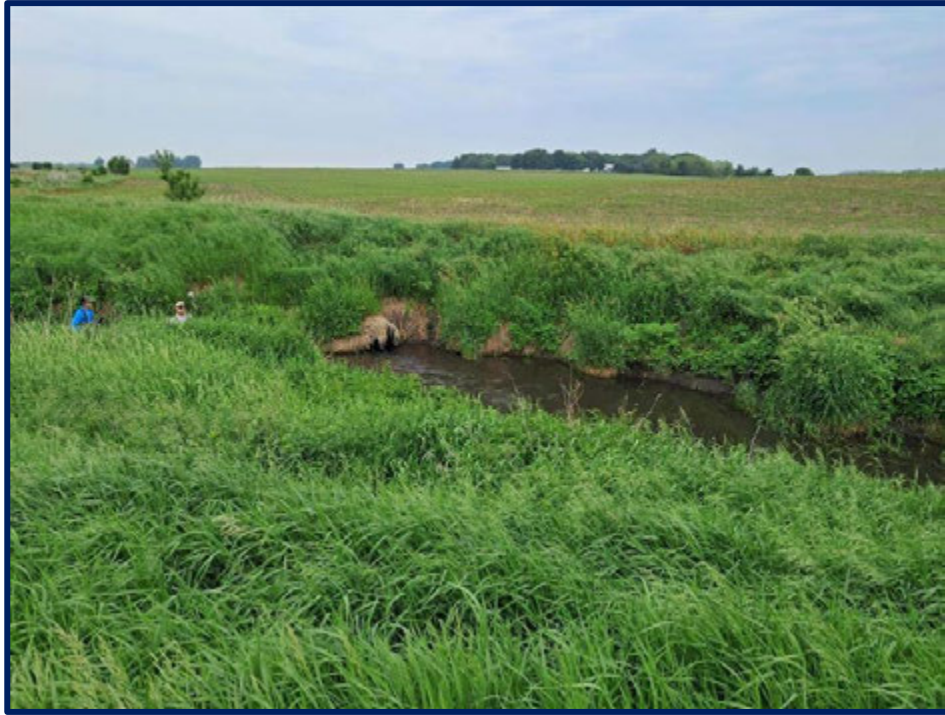
Figure 2. CD 20 Mainline Tile Outlet into CD 12
