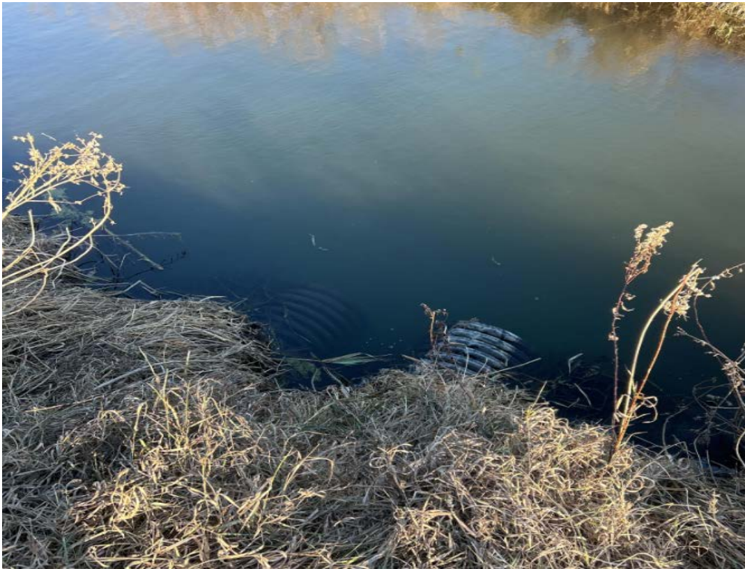
Figure 6. CD 20 Mainline Tile Outlet into CD 12 (NW ¼ of SE ¼ of Section 7 of Delhi TWP)
