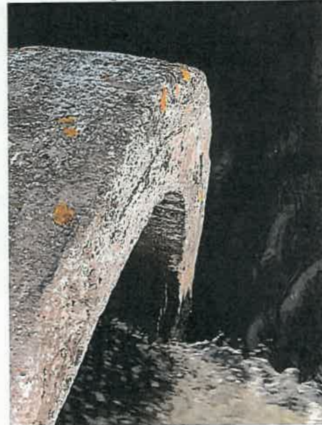
Reinforcement starting to show at end of conduit – Epoxy.
