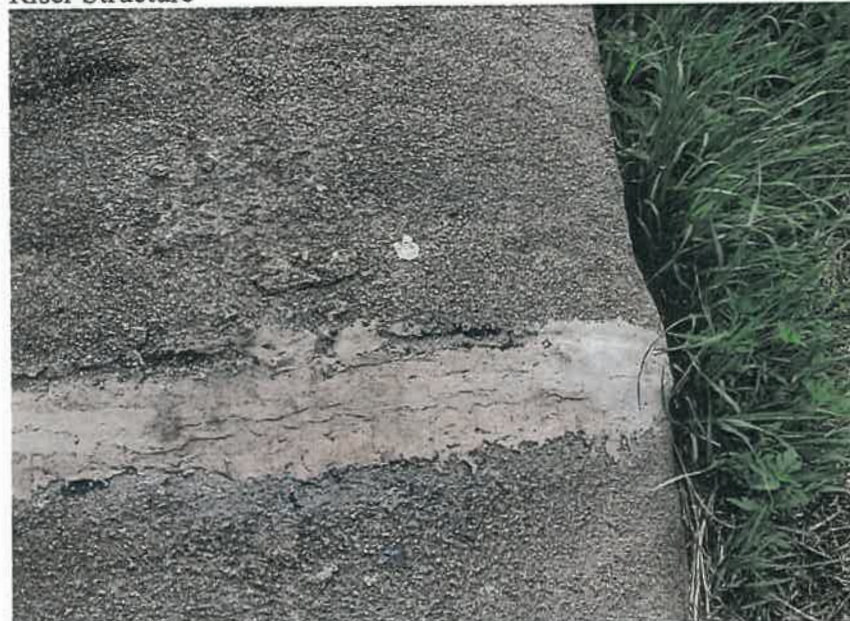
First joint in outlet pipe – small cracks forming – Epoxy
